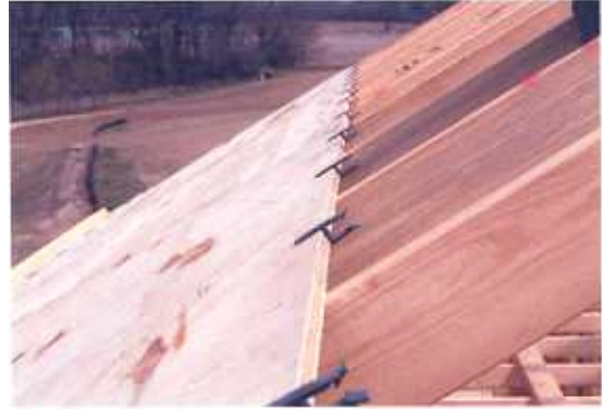
Loaded and ready for the next sheet
